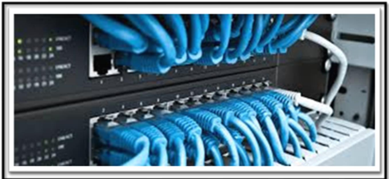
Figure 5-2: Server equipment supplied to Zanzibar Housing Corporation (ZHC) to enhance their IT infrastructure and network operations.
